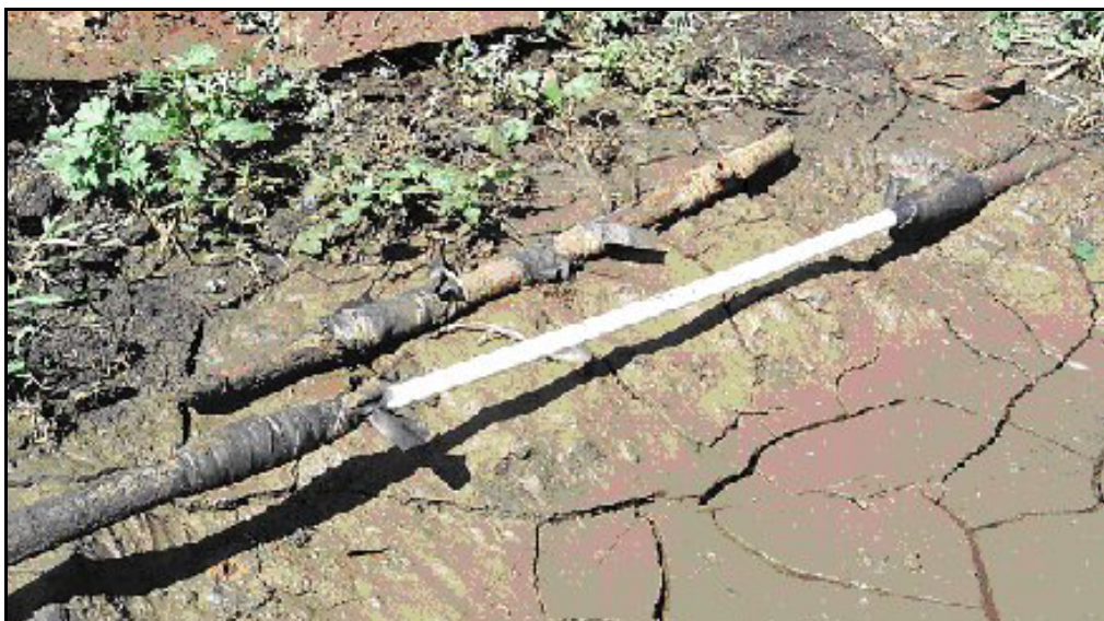
Figure 14 Leakage from village water supply mains repaired with bicycle tubing (TWB photo)
