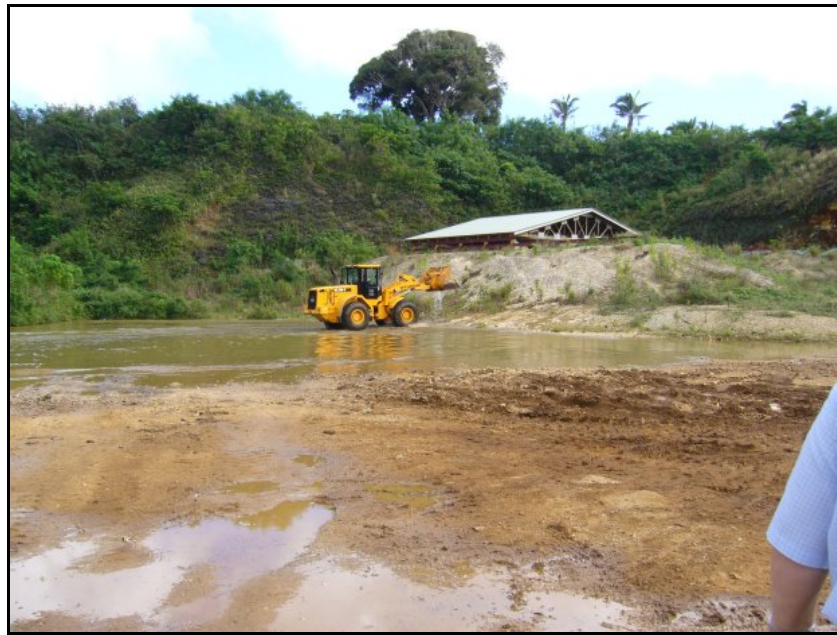
Figure 161 Groundwater exposed at the base of the TWMF being used to wash front-end loader
